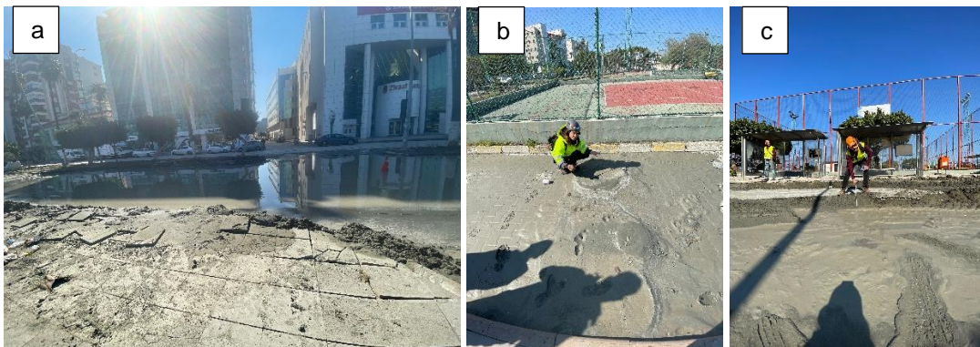
Figure 3-6 Liquefaction manifestations on Ataturk Boulevard near Tennis Courts (~ 36°35'26.95"N/ 36° 10'28.39"E): a) water accumulation and sand boils; b) sand boils; c) ground settlement.
