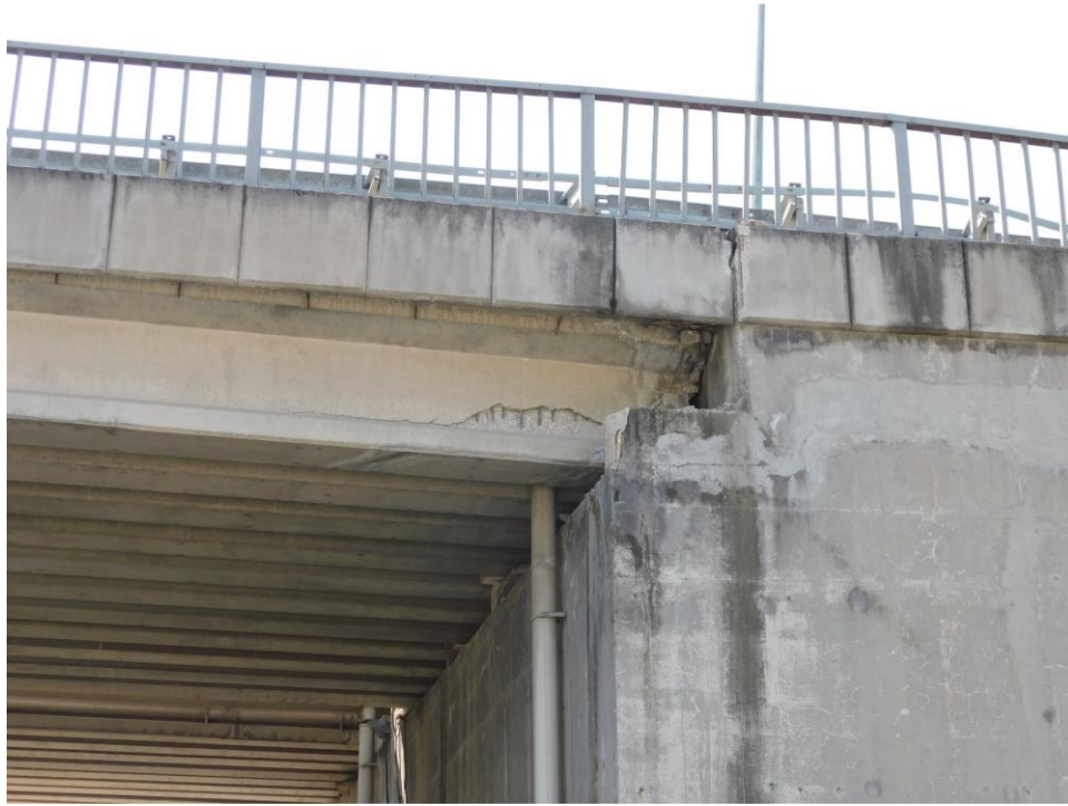
Figure 5-34 Damage at end of Bridge 3 precast girders
