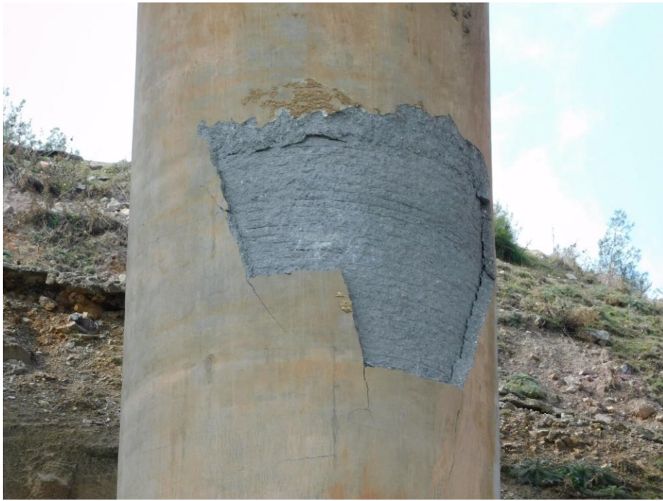
Figure 5-10 Close-up view of column plastic hinge, spalling of cover concrete (opposite side to where vertical bars had buckled), Bridge 1
