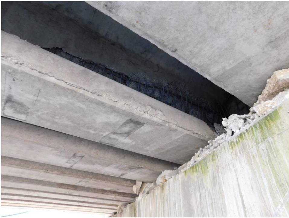
Figure 5-23 Interior girder damage at end of precast girder, Bridge 2
