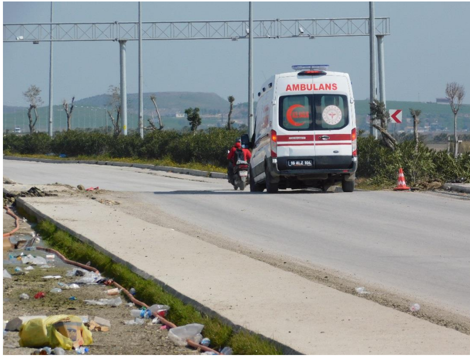
Figure 5-31 Settlement of approach to bridge, View 2, Bridge 2
