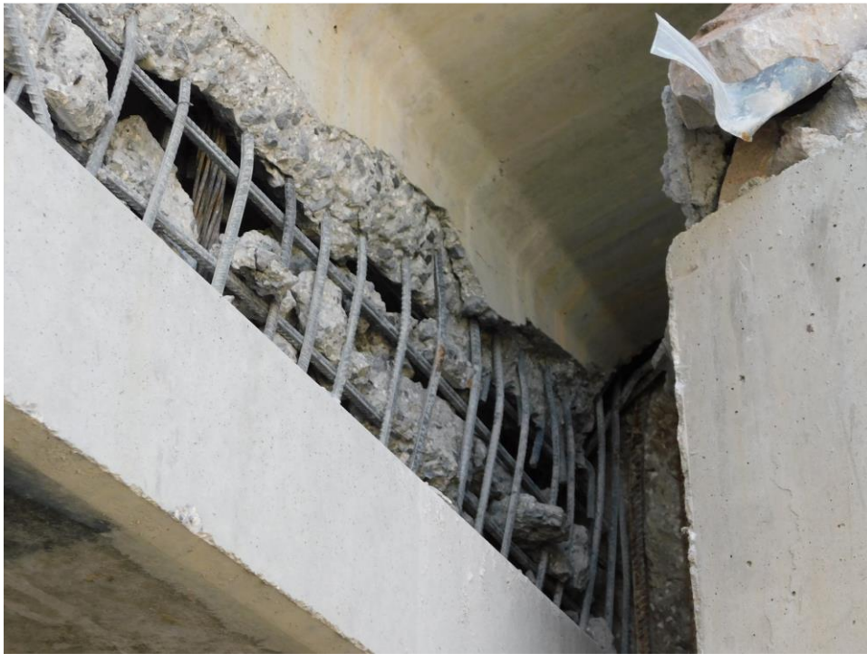
Figure 5-19 Closer view of damage to end of precast girder, Bridge 2
