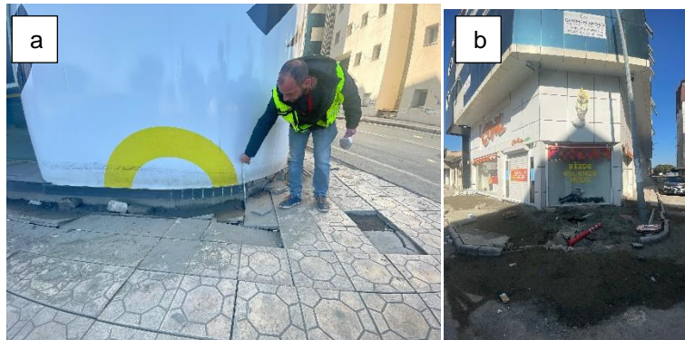
Figure 3-7 Liquefaction manifestation): a) Odeo Bank corner: sand ejecta and liquefaction induced settlements (~36°35'25.92"N/ 36° 10'25.46"E); b) Civilim building corner: sand ejecta (~ 36°35'23.48"N/ 36° 10'23.89"E).
