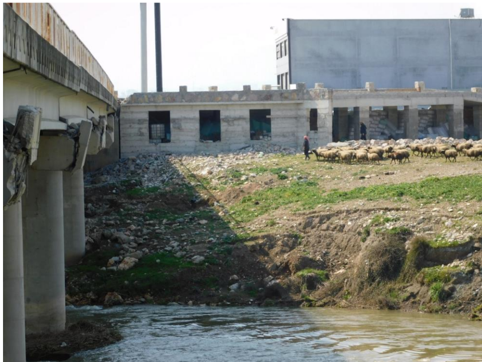
Figure 5-16 Another view of failed exterior shear keys, Bridge 2
