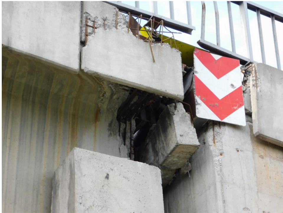
Figure 5-12 Damage at abutment, Bridge 1
