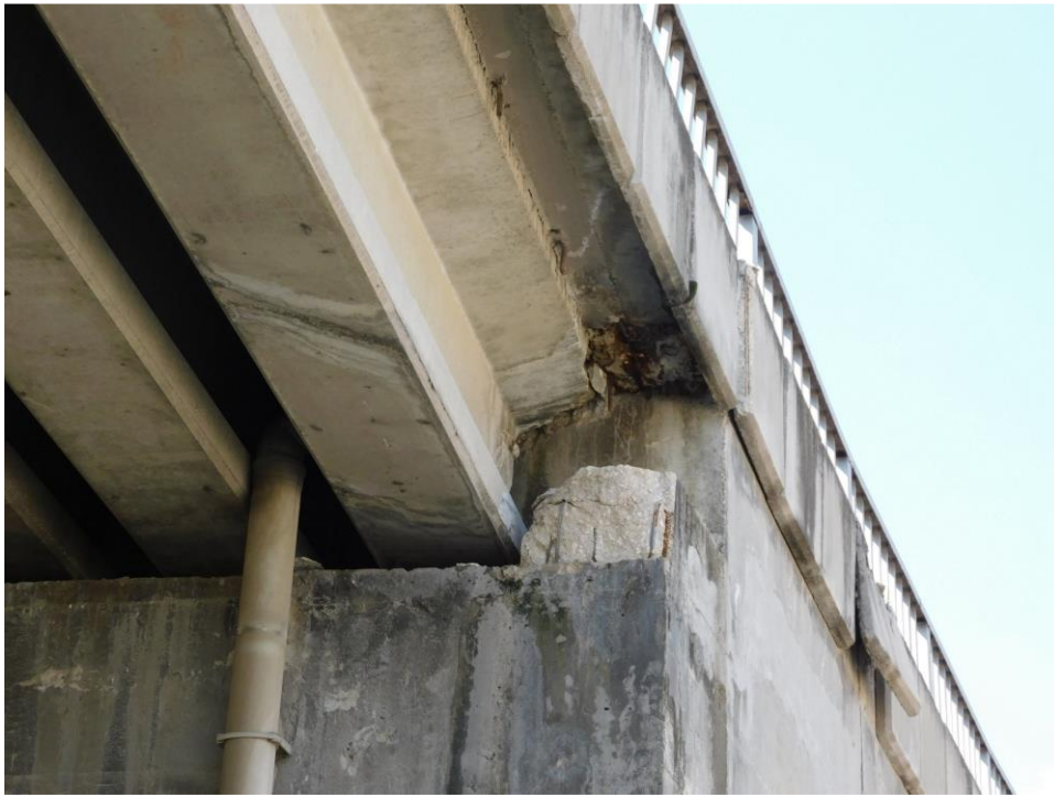
Figure 5-36 Damage of external shear key at Bridge 3 abutment
