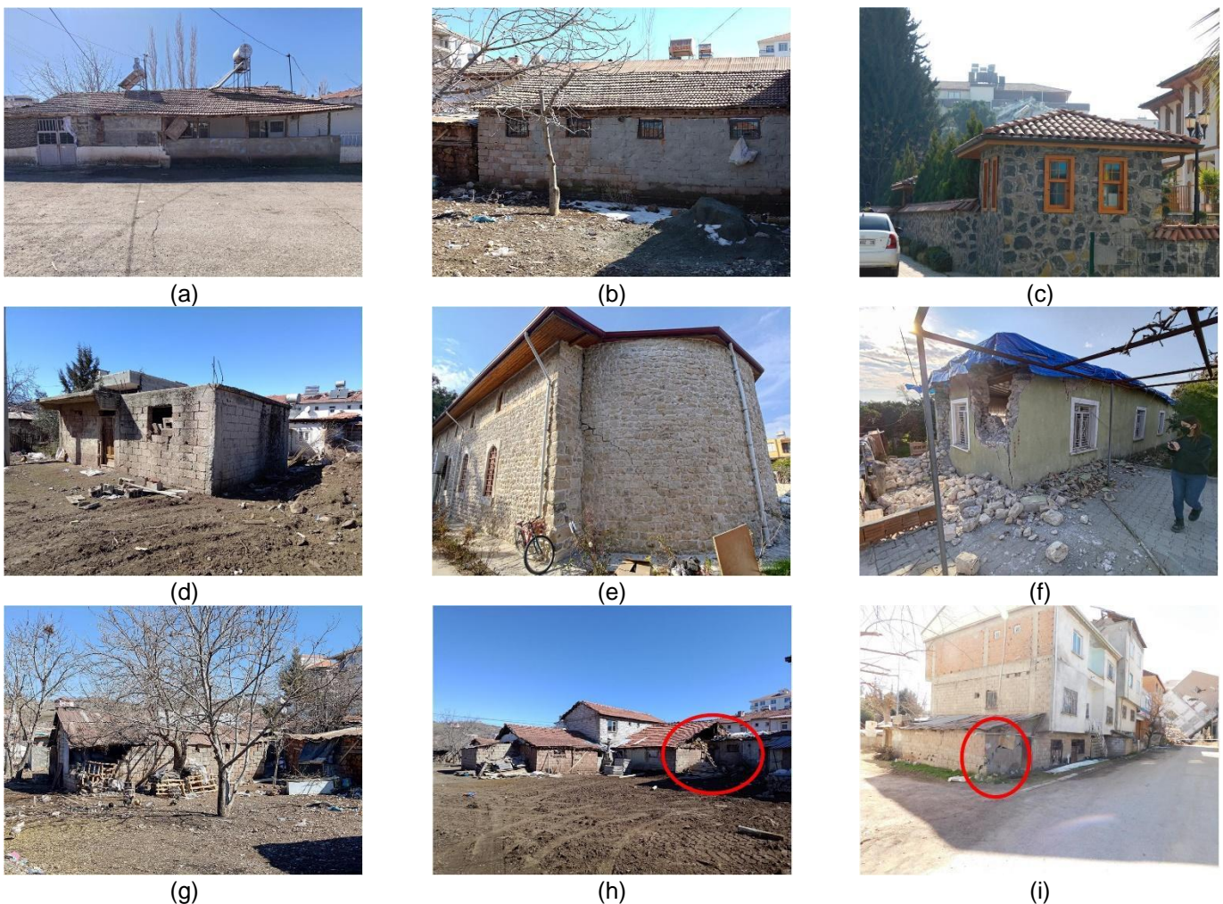
Figure 4-9 (a) to (c) essentially intact or slightly damaged masonry buildings, (d) and (e) moderately damaged masonry buildings, (f) to (h) severely damaged masonry buildings, (i) a pure sliding mode of failure mechanism of a brick wall.
