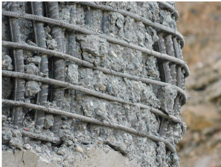
Figure 5-9 Close-up view of column plastic hinge, with buckled vertical rebar and yielded transverse rebar, Bridge 1
