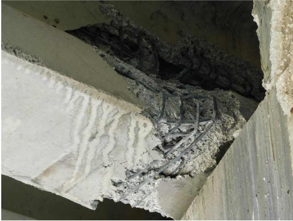
Figure 5-27 Closer view of significant interior girder damage at end of precast girder, Bridge 2
