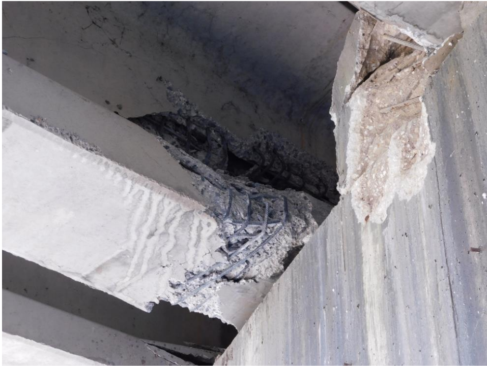
Figure 5-26 Significant interior girder damage at end of precast girder, Bridge 2
