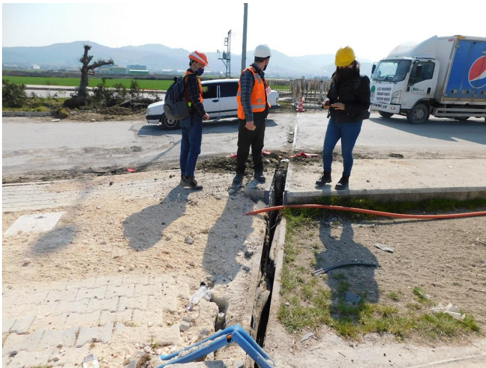
Figure 5-30 Settlement of approach to bridge, View 1, Bridge 2
