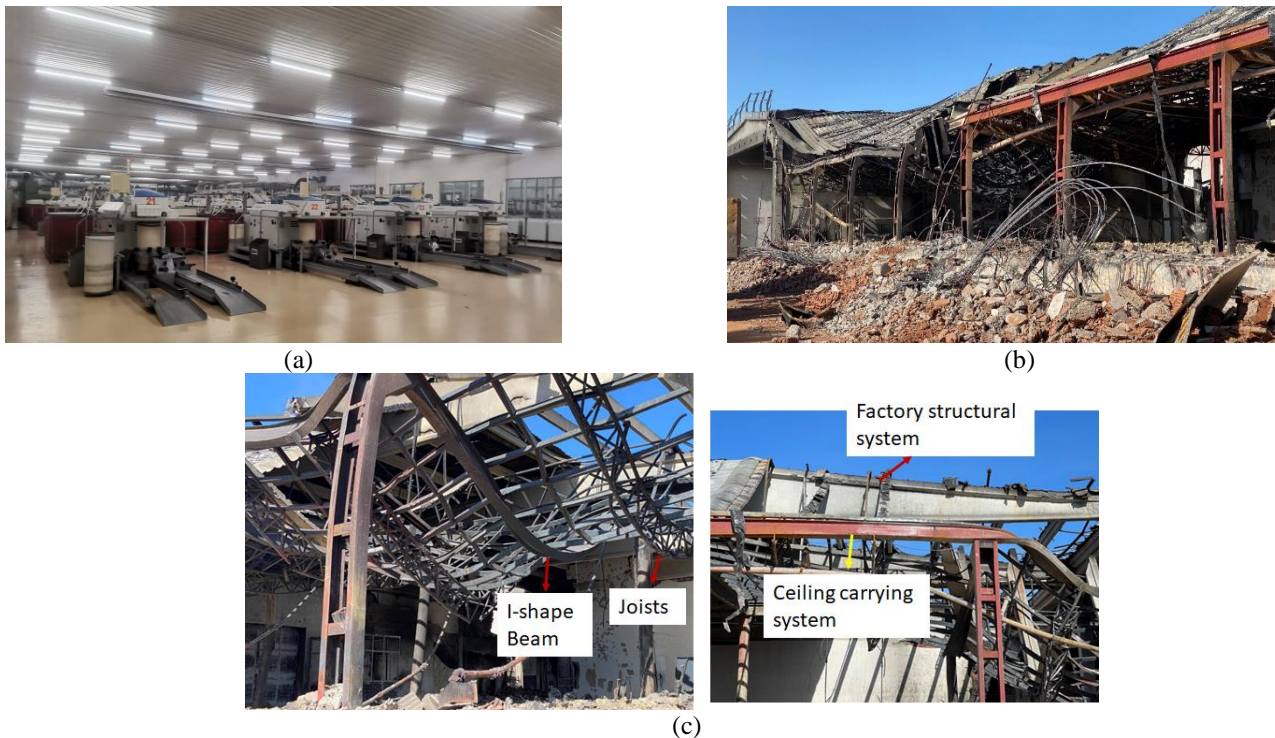
Figure 6-6 Multi hazard on steel suspended ceiling structural system (a) Prior to earthquake, (b) After the earthquake and fire, (c) Detailing
