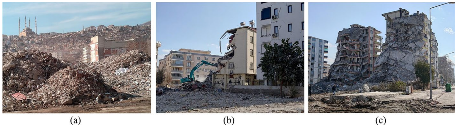
Fig. 15 a Demolition work, b an excavator pulling down damaged buildings, c the damage states of buildings possibly contaminated by demolition work
