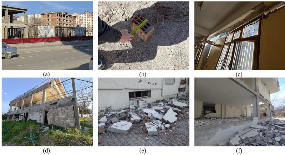
Fig. 20 a Two buildings of one construction project, b a typical brick, c and d brick walls popped out of frames, e brick walls fallen down, f beams and columns were almost intact but brick walls seriously cracked
