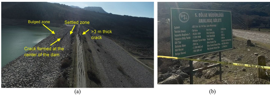
Fig. 10 Deformations observed on the Ariklikas (~37°09′25.70″N/36°30′55.96″E) dams: a Ariklikas Dam (side view); b Ariklikas dam construction details (in Turkish)
