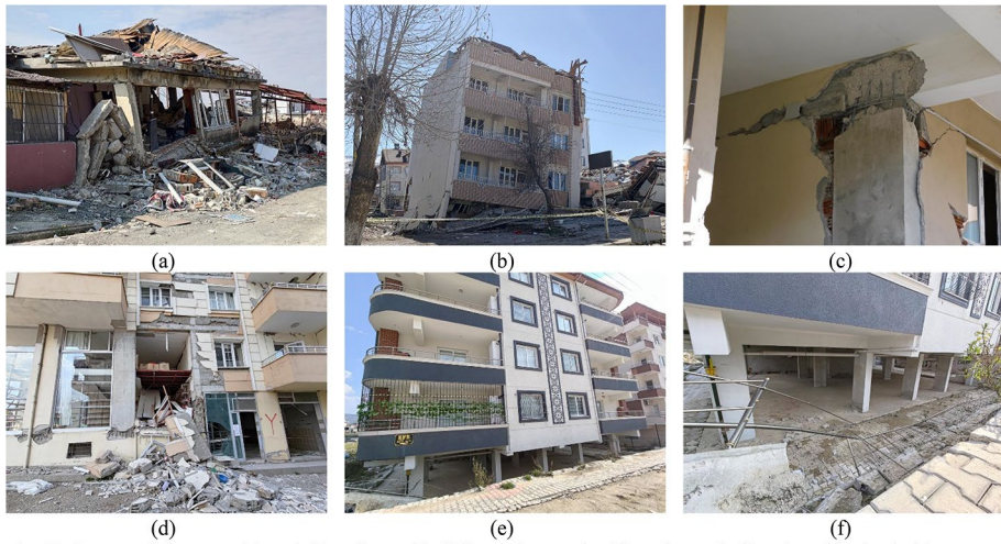
Fig. 19 Structural damages a and b collapsed buildings along a significantly weak direction; c plastic hinges at top and d plastic hinges at bottom of columns, e an almost intact building, and f a close-up photograph of e
