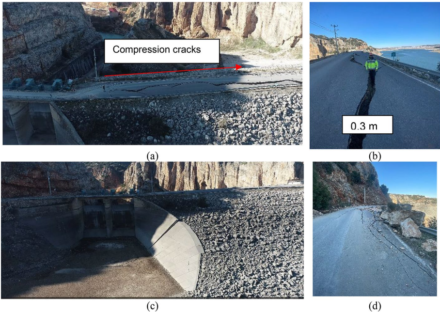
Fig. 9 Deformations observed on the Kartalkaya dam (~37°28′06.01″N/37°14′20.14″E): a compression cracks and lateral displacements at the crest of Kartalkaya dam; b longitudinal cracks in the middle of the crest; c moved segment and compression; d earthquake-induced rock fall and associated cracks on the crest
