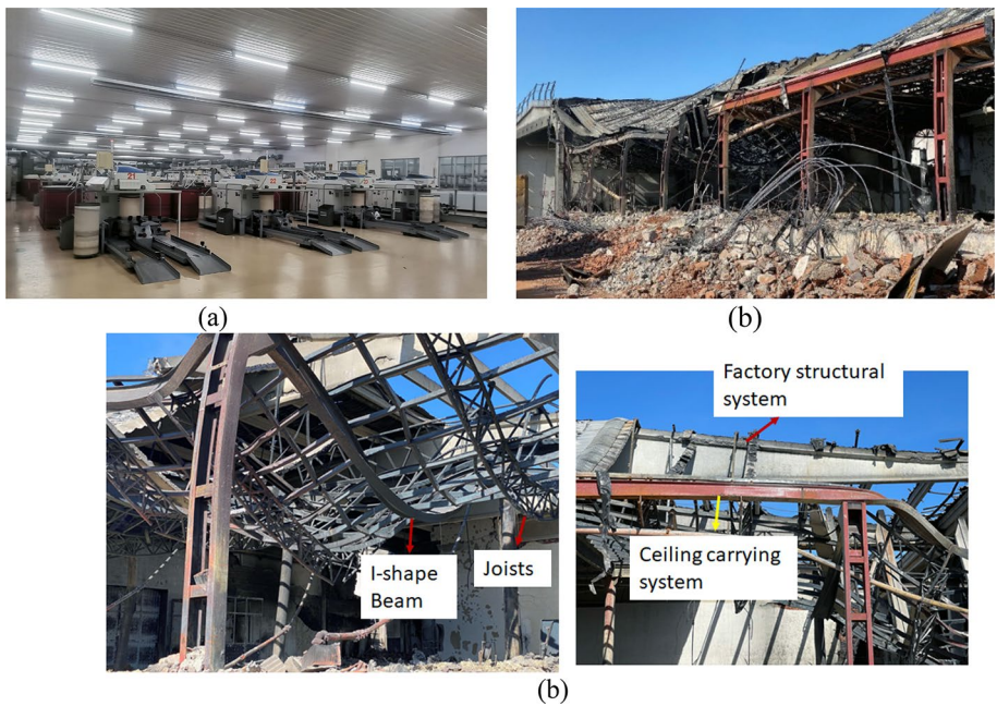
Fig. 33 Multi-hazard on steel suspended ceiling structural system a prior to earthquake, b after the earthquake and fire, c detailing
