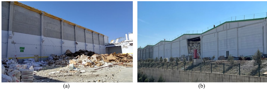
Fig. 30 Damage of precast buildings in Turkoglu OIZ a precast tapered beam failure owing to the loss of support, b cladding panels due to panel-to-structure failure
