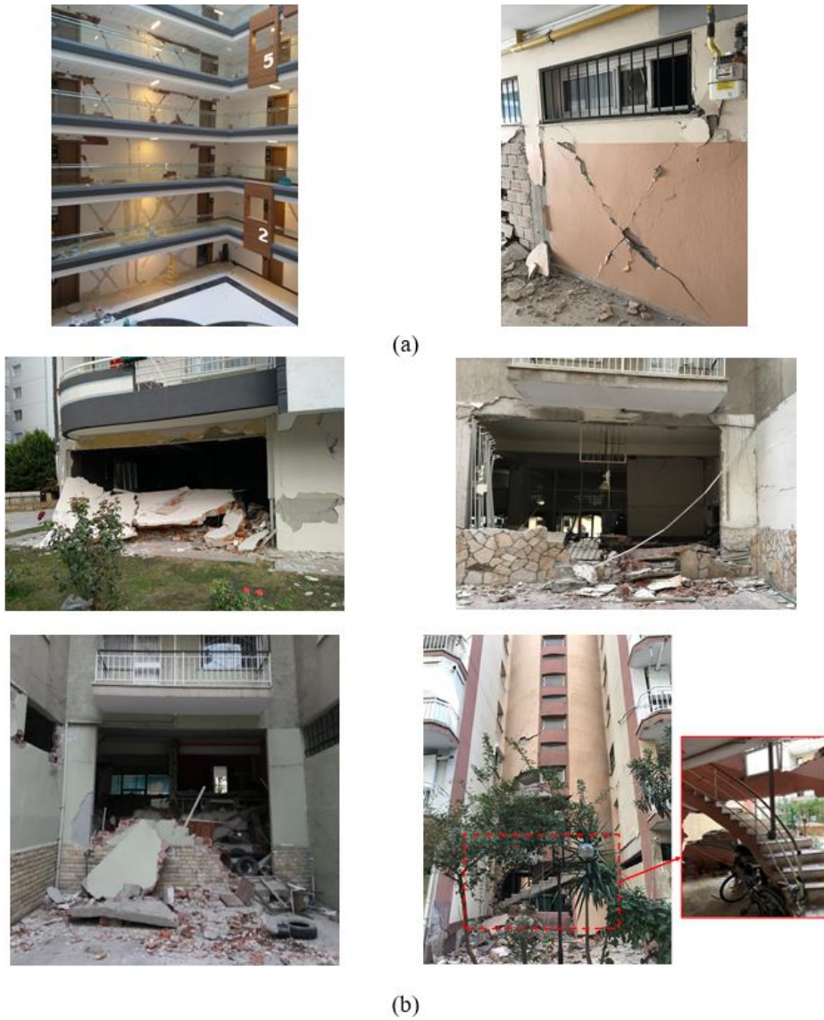
Figure 16. Damage of Infill Walls
