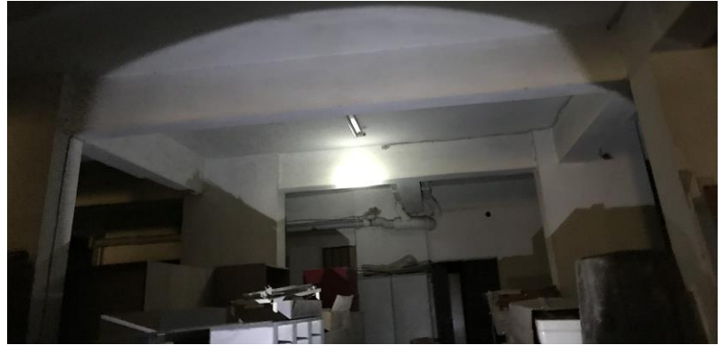
Figure 22. Frame Deficiencies and Irregular Floor Layout
