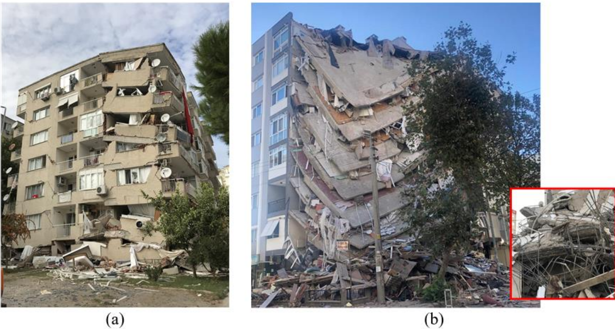
Figure 12. Partially Collapsed Building, Located at the Street Corner
