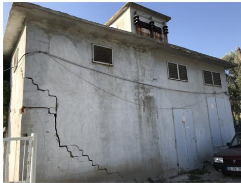
Figure 23. Damage at the corner of the masonry power distribution unit
