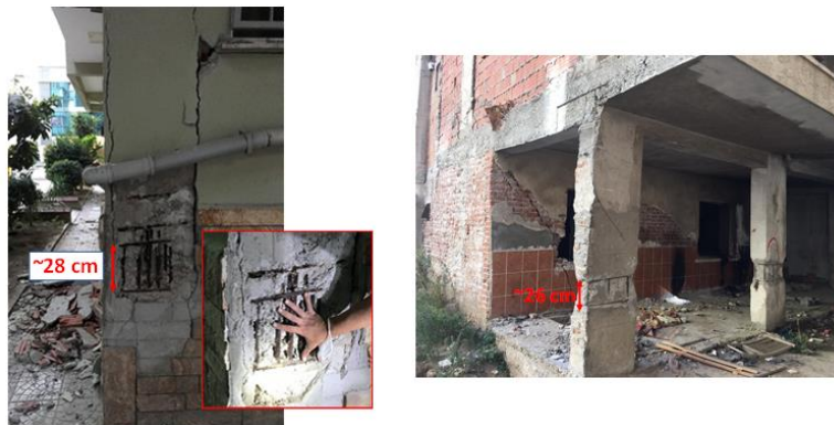
Figure 19. Inappropriate Reinforcement Spacing and Excessive corrosion in the reinforcement
