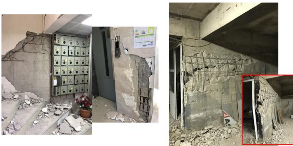
Figure 17. Buckling of Distributed Vertical Reinforcement in Shear Walls
