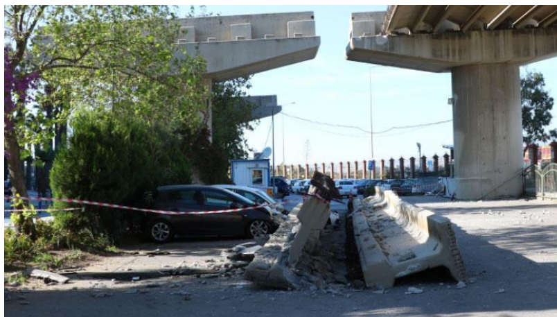
Figure 30. a) Girder fall from unfinished bridge viaduct construction in Alsancak due to no lateral connection detailing (Photo is adapted from https://i4.hurimg.com/i/hurriyet/75/0x0/5fa6a9f00f254410e87185f2 )
